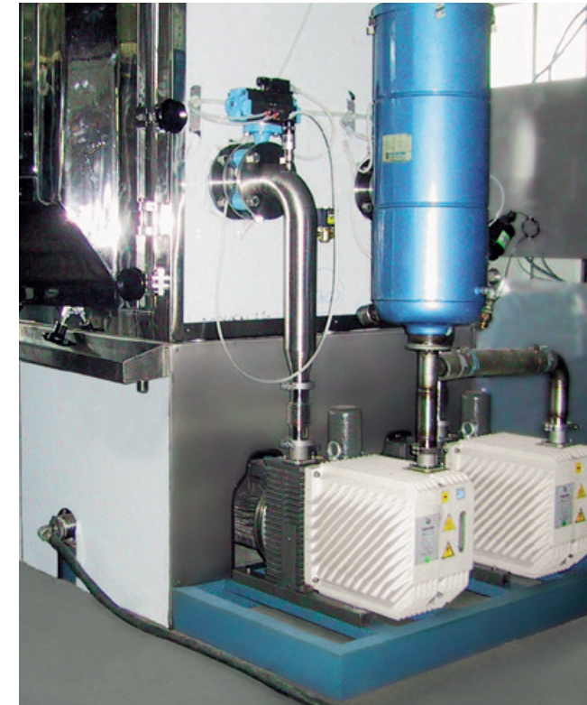
Freeze Drying equipment.
